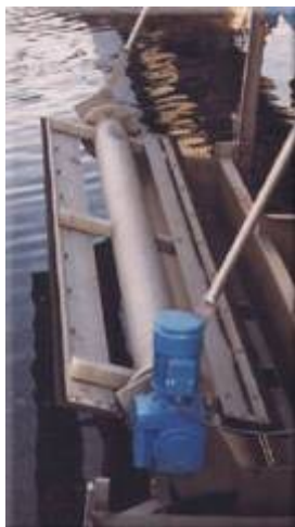
Wastewater systems – agitator – aerator Low speed Humid & moist environment
